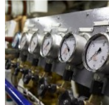
Process control system
